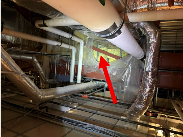
FIGURE 20 TORN VAPOR BARRIER
