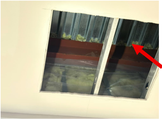
FIGURE 7 TYPICAL CONDITION ABOVE BUMP-OUT ON THE NORTH WALL
