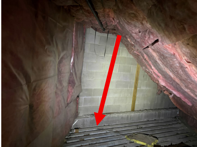
FIGURE 14 INTERIOR OF DORMER AT LEAK #2
