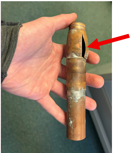
FIGURE 2 FROZEN PIPE REMOVED
