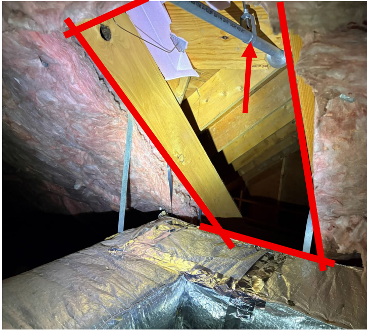
FIGURE 2 (2' X 6') HOLE TO ENTRY DORMER W/ SPRINKLER PIPE
