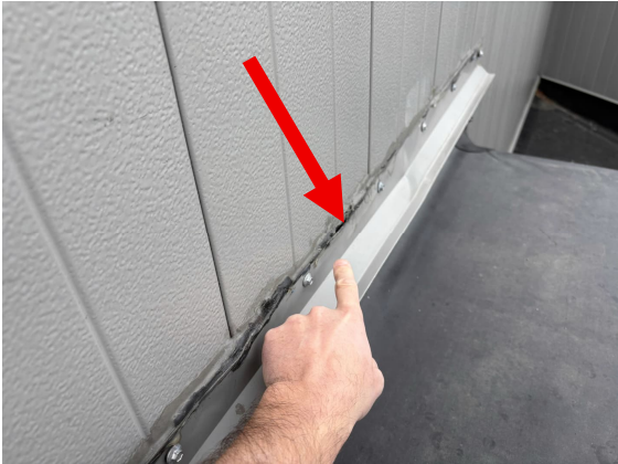
FIGURE 12 BROKEN SEALANT JOINT
