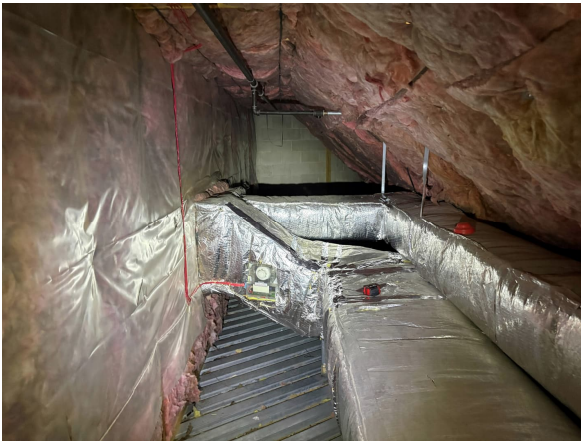
FIGURE 5 HARD TO REACH DUCTWORK ABOVE THE ENTRY
