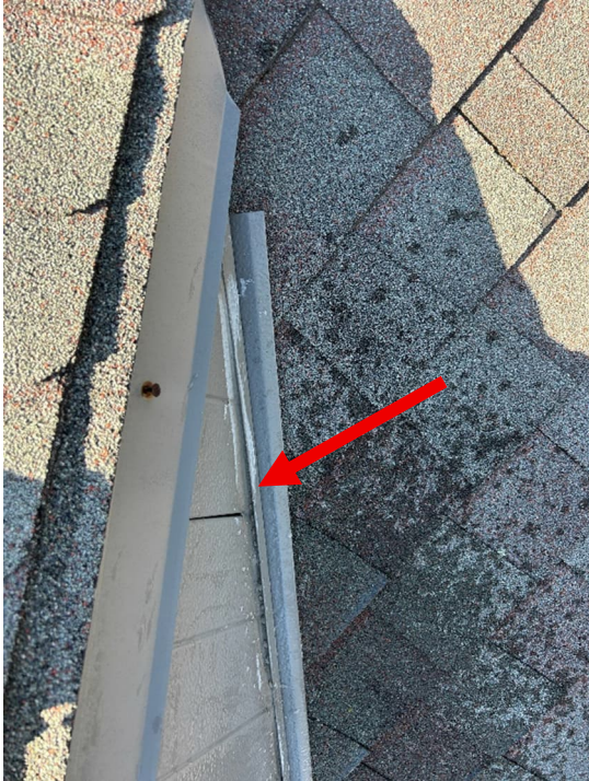
FIGURE 13 LEFT SIDE OF DORMER (HIGH): LEAK #2
