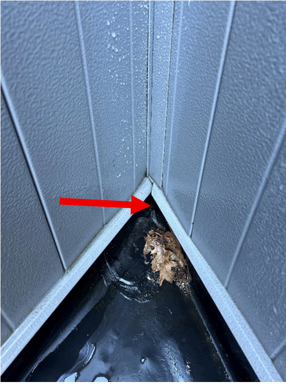
FIGURE 4 LOCATION OF LEAK #1 IN RIGHT CORNER
