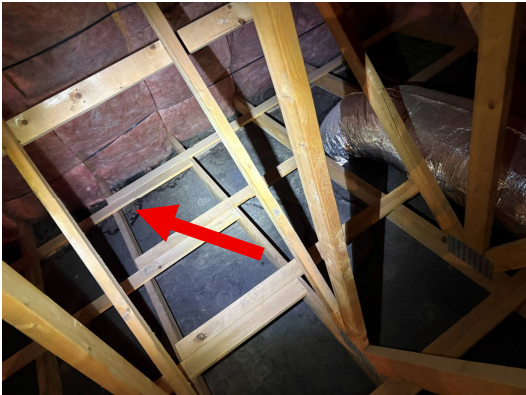
FIGURE 14 WATER STAINING AT NW CORNER OF CHILDREN'S READING ROOM
