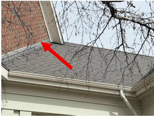
FIGURE 9 MISSING SELANT JOINT
