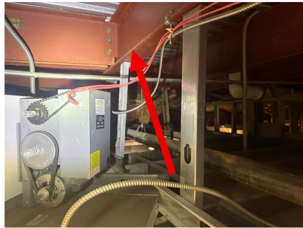
FIGURE 4 WATER STAINING ON STRUCTURAL BEAM
