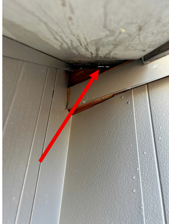
FIGURE 17 UNDERSIDE OF SOFFIT AT LEAK #2
