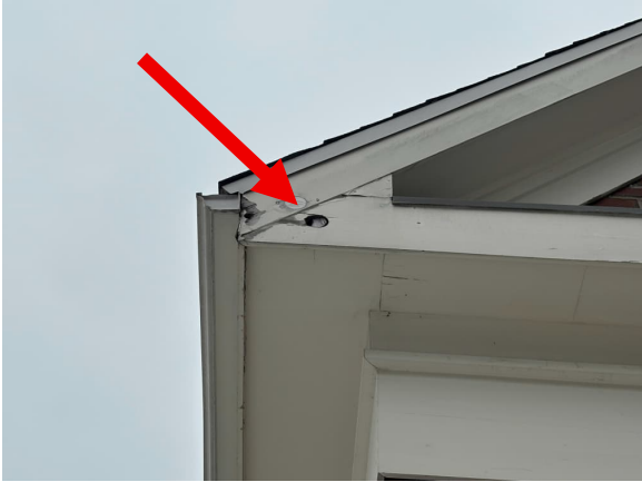
FIGURE 21 TYPICAL PAINT AND PATCH REQUIRED
