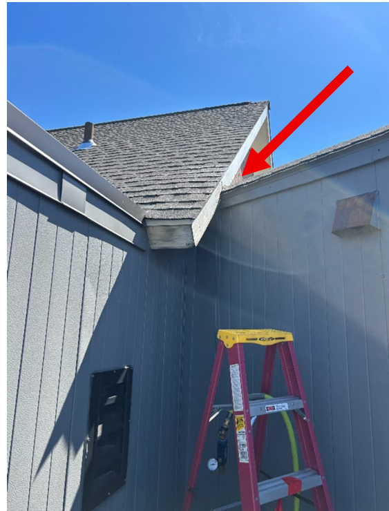
FIGURE 12 LEFT SIDE OF DORMER (HIGH): LEAK #2
