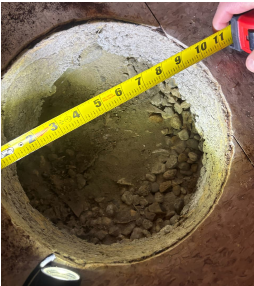
FIGURE 11 EXPLORATORY HOLE OBSERVED
