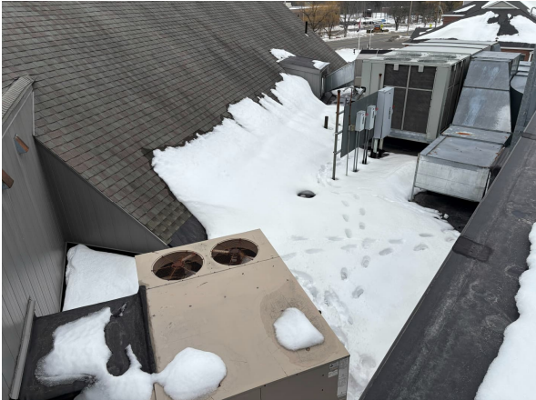
FIGURE 15 ROOF TOP EQUIPMENT
