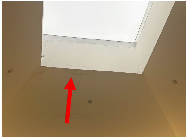
FIGURE 17 WATER DAMAGE AT SKYLIGHT
