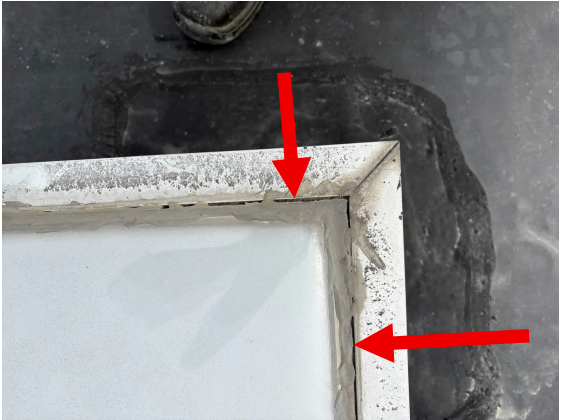
FIGURE 13 BROKEN SEALANT JOINTS
