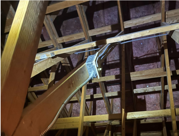
FIGURE 12 APPEARS THAT THE VAPOR BARRIER IS MISSING
