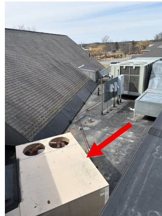
FIGURE 6 AHU #3 ON OTHER SIDE
