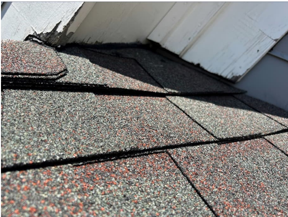
FIGURE 15 INSUFFICIENT SPACE BETWEEN MATERIALS.
