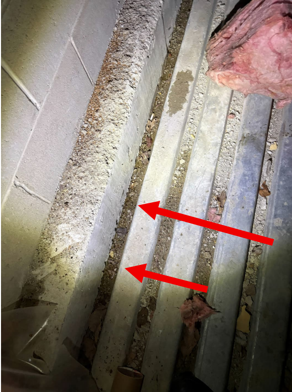
FIGURE 16 WATER BUILD UP IN DORMER FROM LEAK #2
