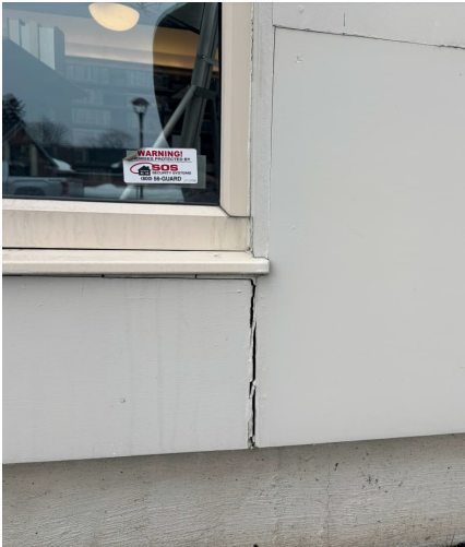
FIGURE 23 TYPICAL PATCH AND PAINT REQUIRED
