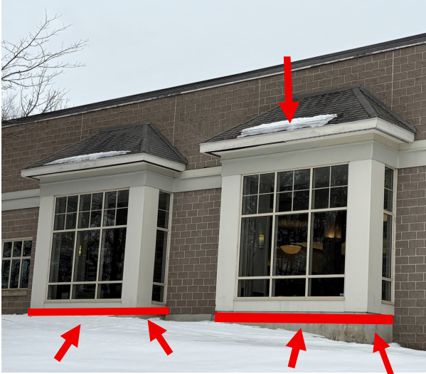
FIGURE 5 MISSING FOUNDATION INSULATION
