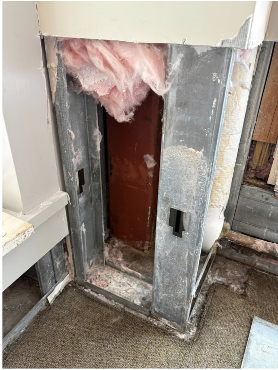
FIGURE 4 COLUMN ENCLOSURE REMOVED AT BASE
