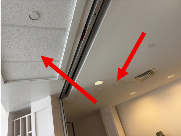
FIGURE 14 AREAS OF PROMINENT LEAKS
